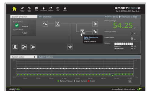
STATUS OF DC/DC CONVERTERS IN SMARTPACK2 WEB
